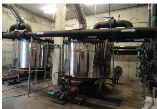
Figure 2. Thermal power plant installed at a Public Health administration building in Mérida (Badajoz).
