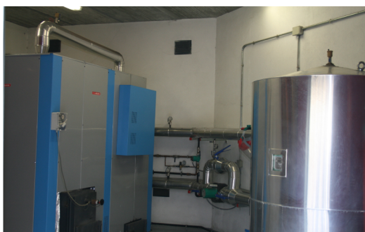
Figure 1. Thermal power plant installed at Zafra Hospital (Spain).
